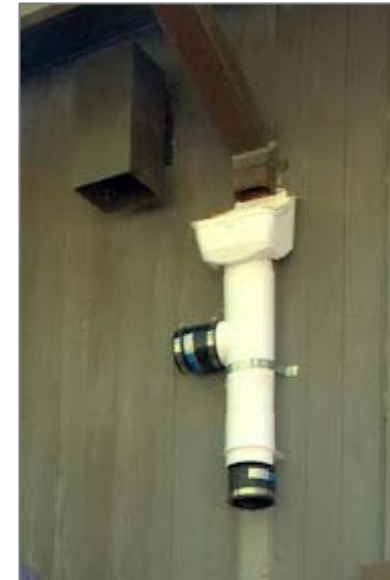
First flush and downspout diverter installation Courtesy of The City of Oakland
