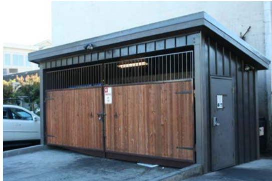
The above enclosure shows a security rail that has been attached to the gates to avoid pedestrian entrance and/or waste deposits over the gate.
