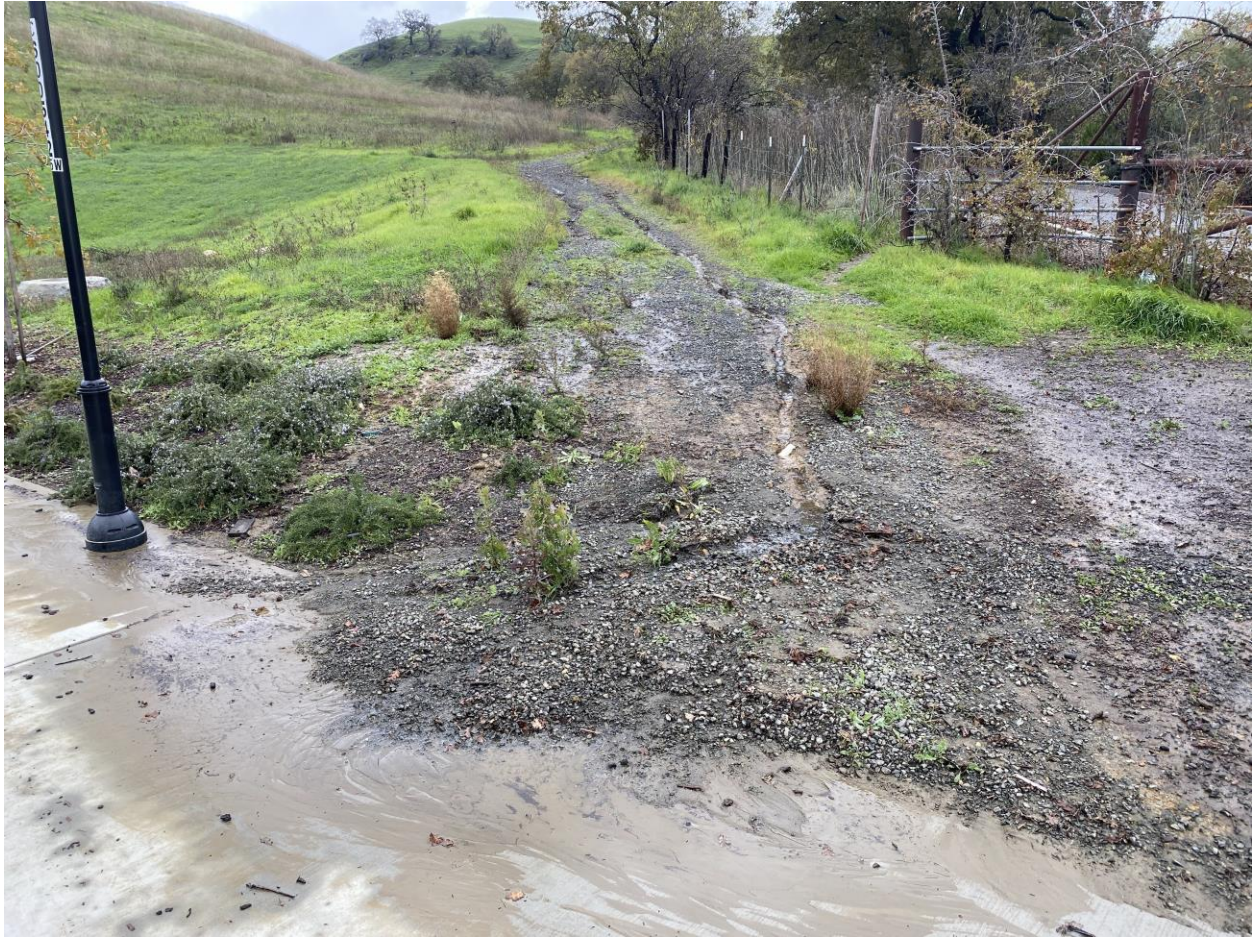
Erosion gully within maintenance road north of Area "L"
