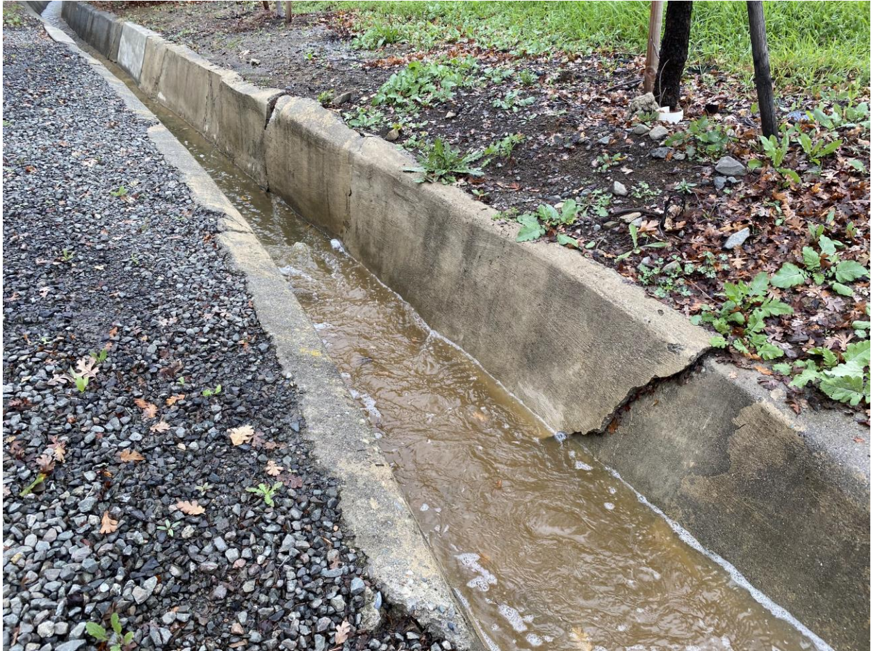
Damaged section of concrete-lined drainage ditch
