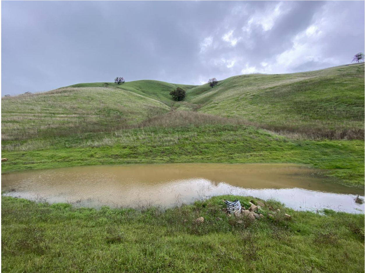
Accumulated sediment partially covering riprap-lined aprons at terminus of swales upslope of Sedimentation Basin "A".
