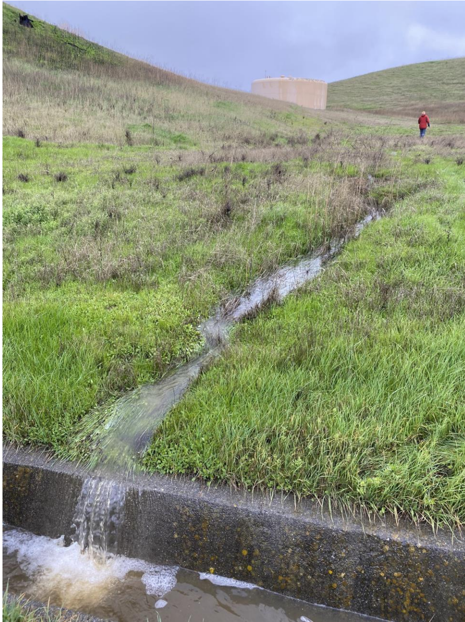
Erosion gully flow discharging into offsite concrete-lined drainage ditch north of Solano Irrigation District Water Reservoir
