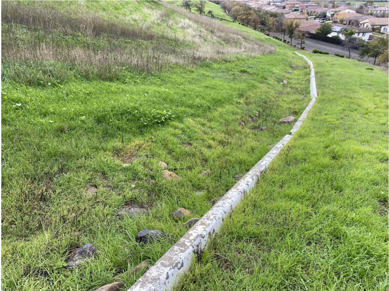
Deflection wall east of Sedimentation Basin "A" filled with soil and vegetation
