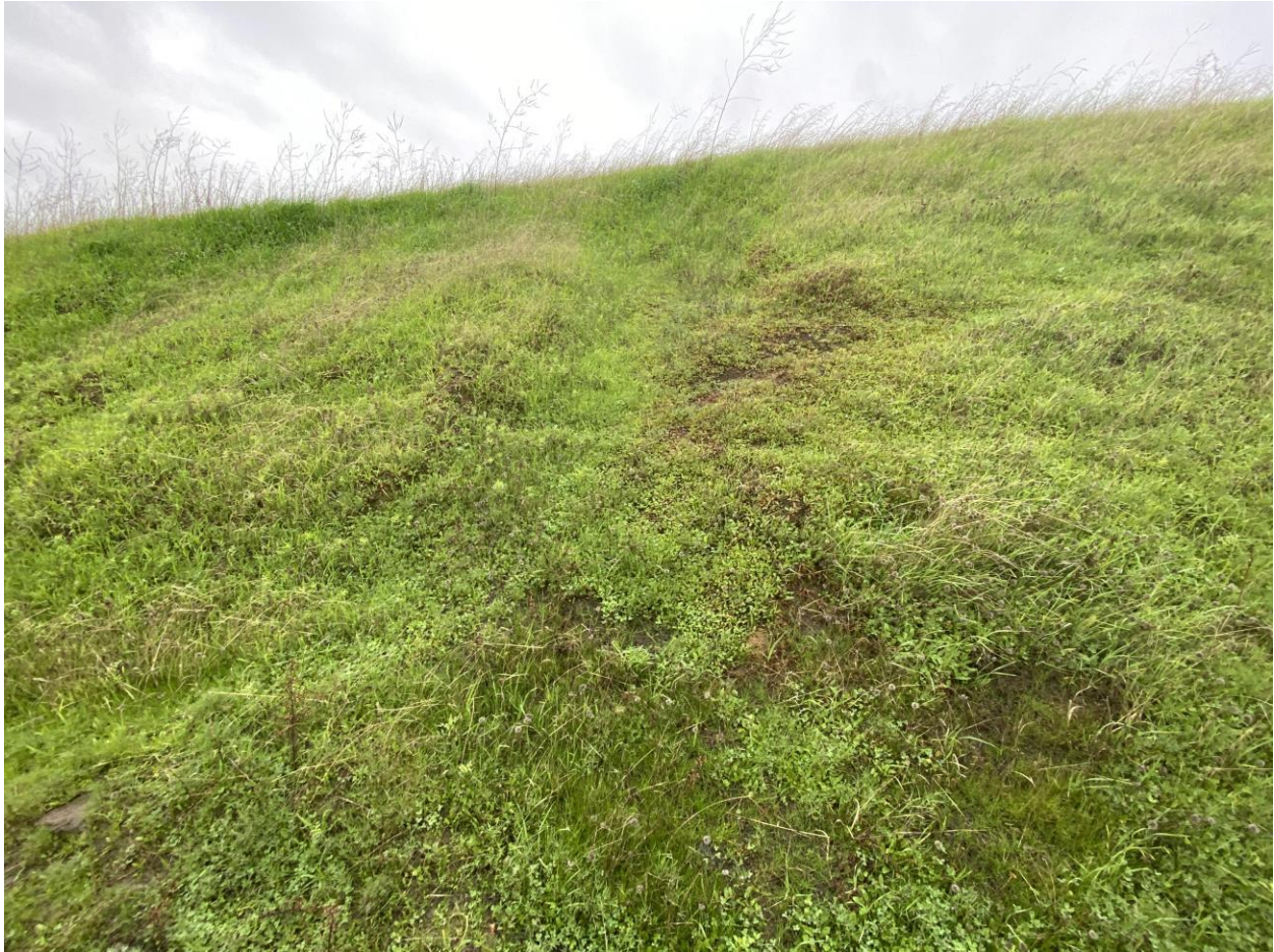
Shallow landslide along embankment near Solano Irrigation District Water Reservoir
