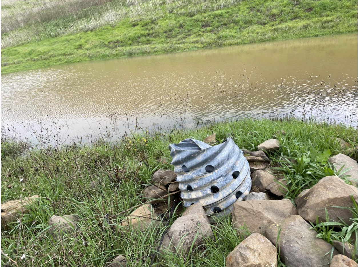
Damaged outlet drainage pipe with missing grate in Sedimentation Basin “A”
