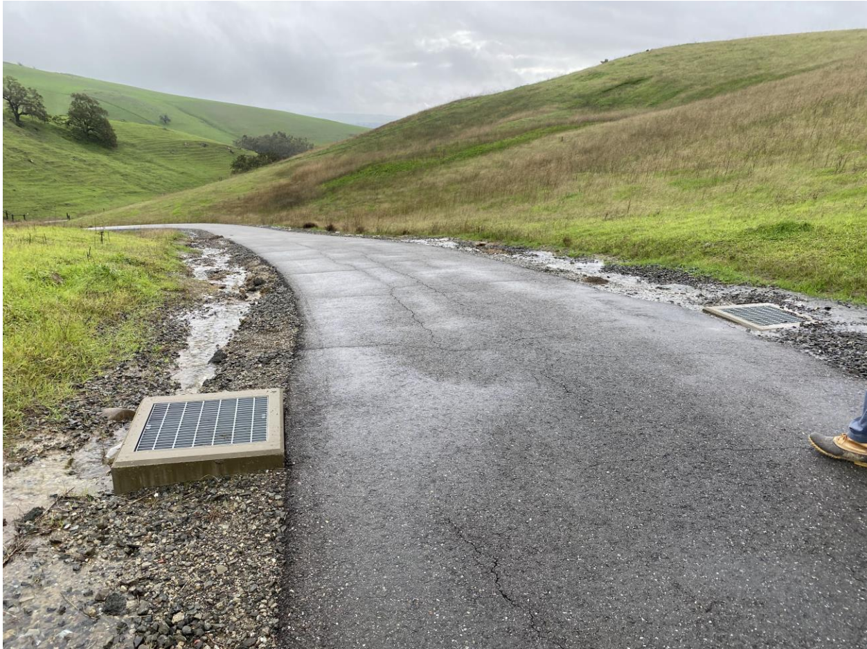
Erosion gullies along paved access road to Solano Irrigation District Water Reservoir
