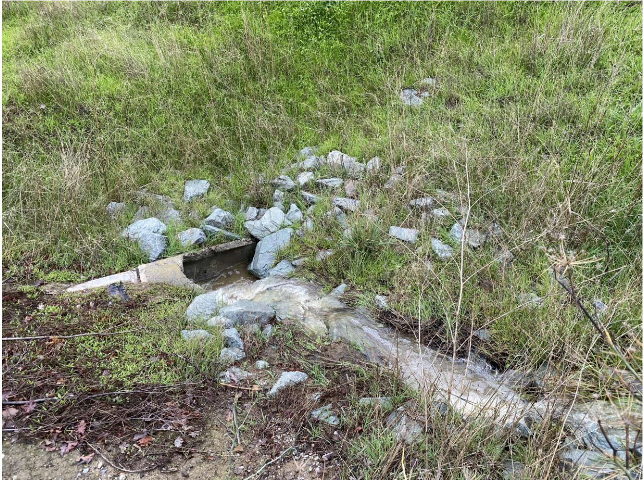
Damaged storm drain pipe along paved access road for Solano Irrigation District Water Reservoir
