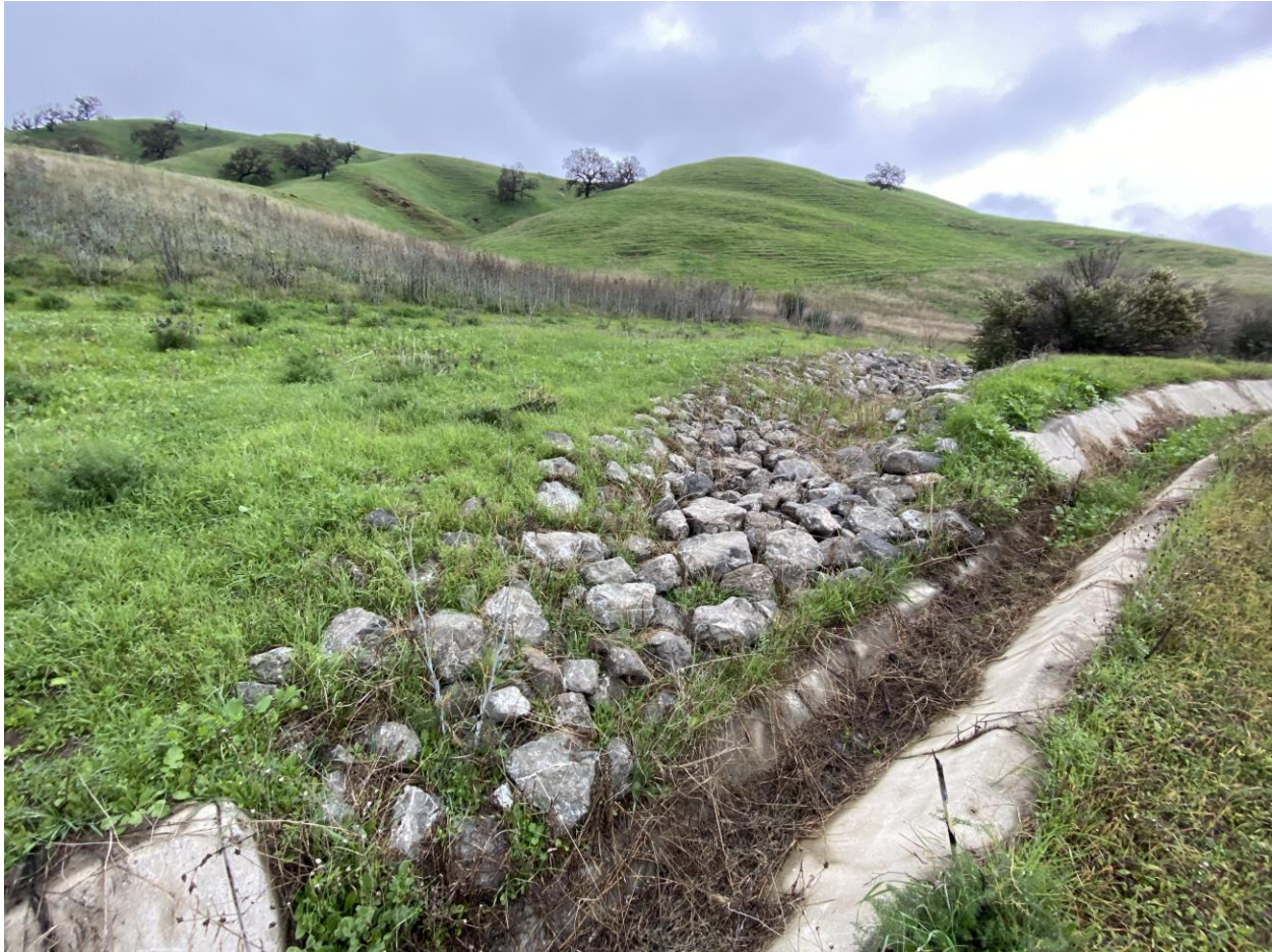
Vegetation growth within riprap outfall apron for Sedimentation Basin "1"
