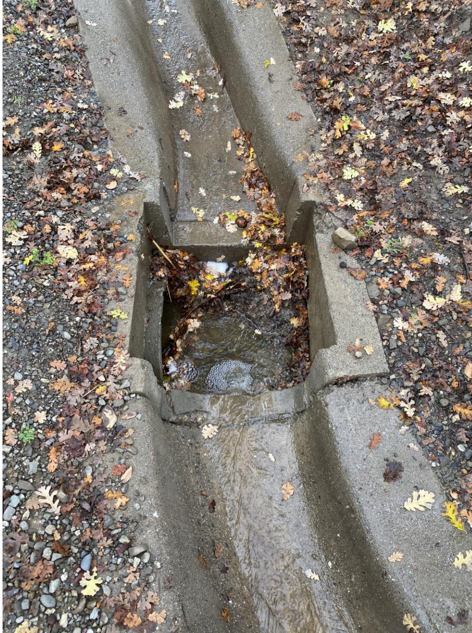
Storm drain inlet with missing grate
